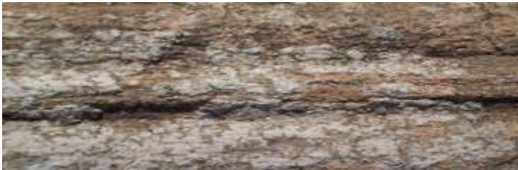
Fig. (16) biodeterioration of plasters.
