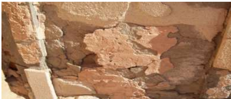
Fig. (17 ) deteriorated of plasters
