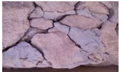
Fig. (10) Deterioration and disintegration of unsuitable mortars .
