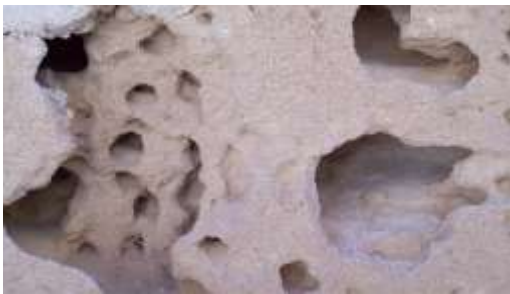
Fig. (9) Erosion of limestone by weathering are the principle factor of honeycomb and damage of limestone
