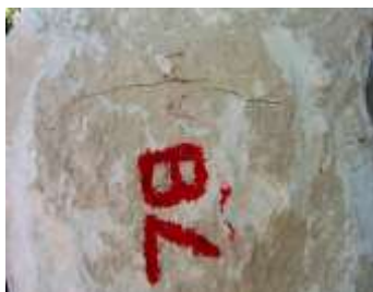
Fig.(6) shows the cracks and microcracks.
